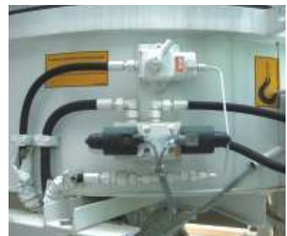
Manual emergency emptying
