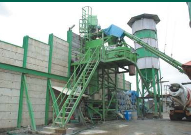
CP 30 Batching Plant working in RMC
